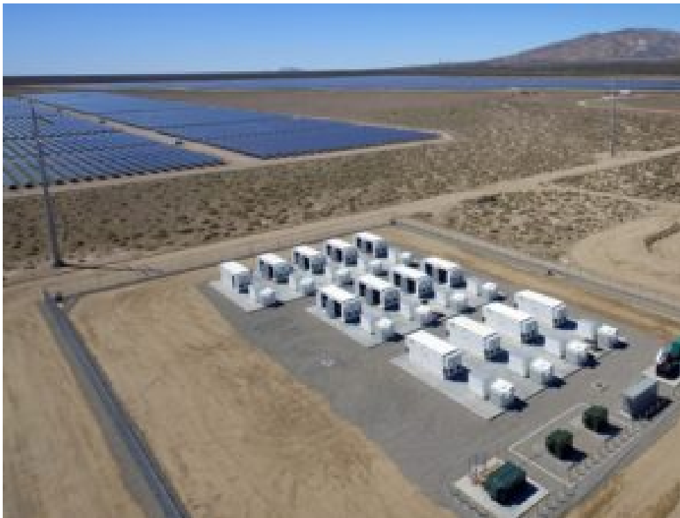
The Beacon BESS now stabilizes and stores energy from Beacon Solar Plant in the Mojave Desert. (Photo by Chris Corsmeier)
