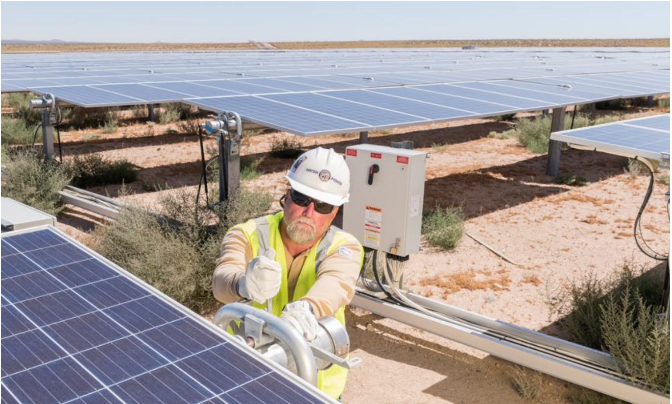
Steve Taylor, Sr. Electrical Craft Helper, works on solar array. (Photo by Chris Corsmeier)
