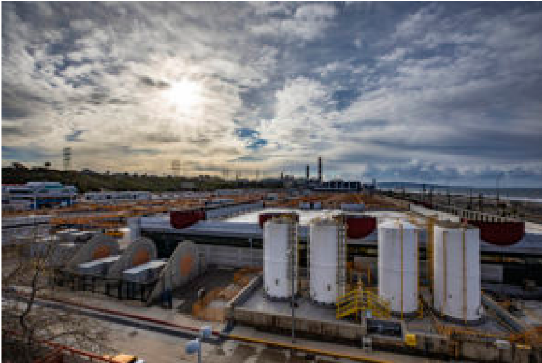
Hyperion Water Reclamation Plant
