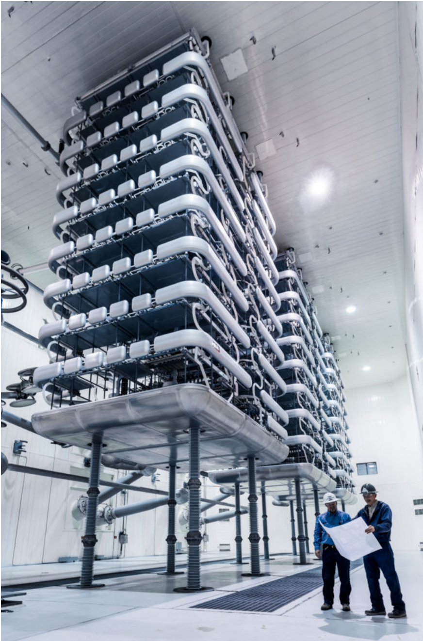
Giant thyristors at Sylmar Converter Station. Photo by Chris Corsmeier
