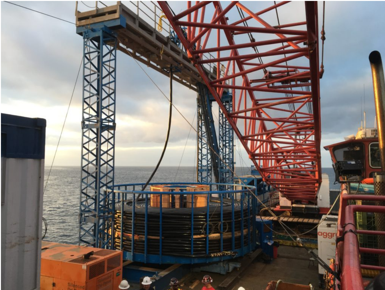
The project included replacing both underground cable on land and submarine cable under 120 feet of water in the Pacific Ocean. (Photo by Jairo Guerrero)
